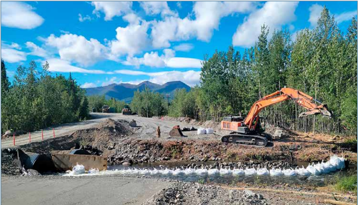
Groundwork began on the Little Tonsina River in 2022 with existing culverts acting as coffer dams for in-channel construction (bed and banks) to take place “in the dry” as much as practicable. Picture from K. Liebich, USFWS.
