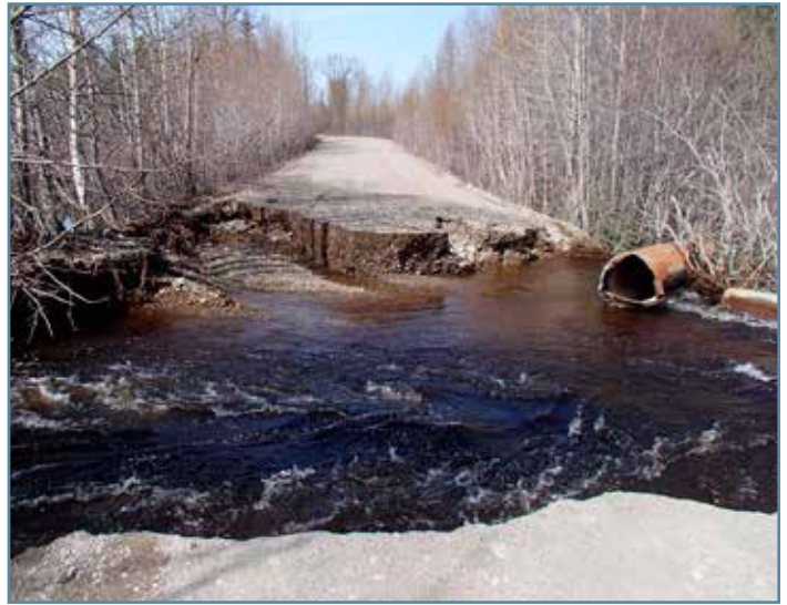
A small round culvert that failed during a 2012 flood event. Photo from USFW.
