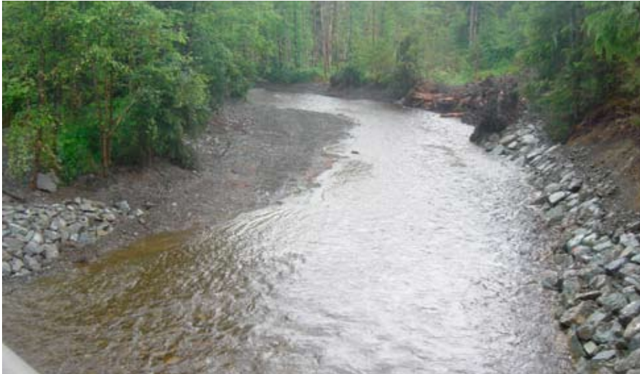
Fubar Creek after Phase I restoration, flowing for the first time in 13 years. (USFS photo).
